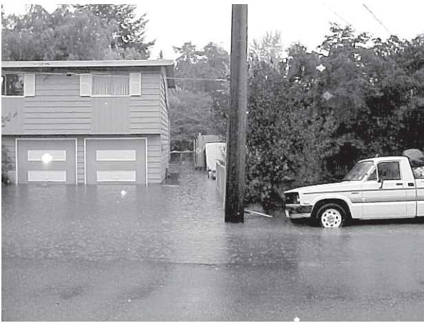
The 3rd Ave. NW Drainage improvement project will provide relief to over 20 homes and local streets from flooding such as occurred during the Oct. 20, 2003, storm.
